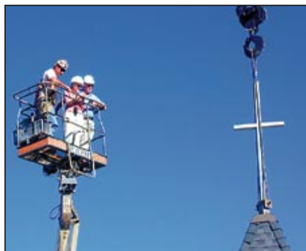
Pat Bedynek, of Dennis Steel, lifts Gayle Cipriano, Co-Building Chair, and Dick West, Covenant UMC Senior Pastor, to get a better view.
