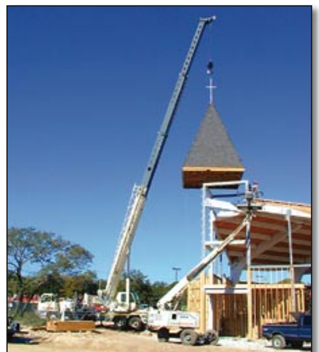
A 60-ton crane from Crocker Crane Rental lifts the 18,000 pound steeple into position at Covenant UMC.
