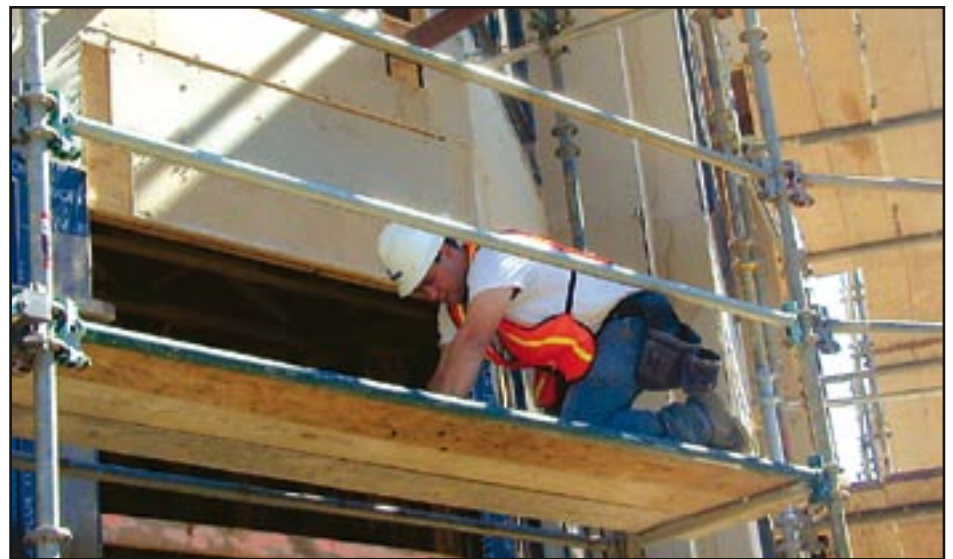
Mike Beasley, of Jordan Construction, measures exterior wall board to hang at 404 Rio Grande.
