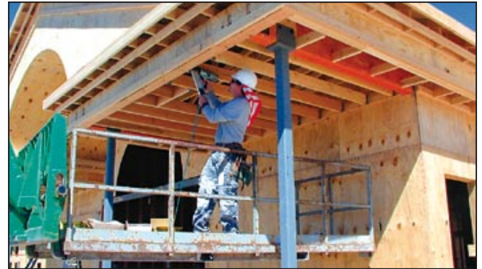
Jeremy Daley of White, Inc., frames an awning for a new LDS church in Pflugerville, built by Bud Bailey Construction.
