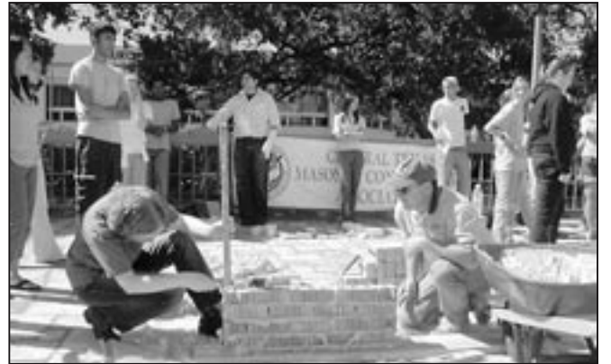
Chris Toth of CD Lonestar, Inc., keeps a level head as he instructs UT Architecture students at Masonry Day.
